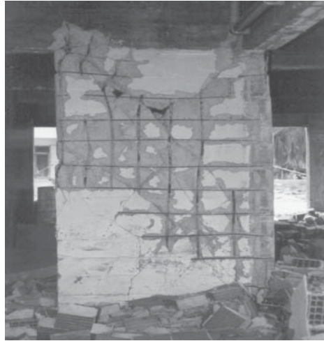
Shear wall after an earthquake. Courtesy of Murat Saatcioglu and John Gardner
